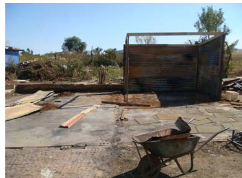
What was left of Rainbow Day Care Centre after the theft and fire
